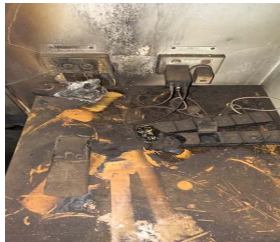
Figure 2: Li-ion power bank fire in village room
